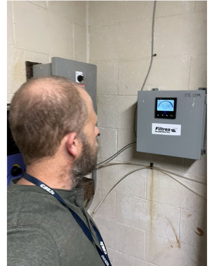
Photo depicts Public Health Sanitarian, Eli Rust, conducting an inspection of the flow meter for the filtration system of a swimming pool facility.
